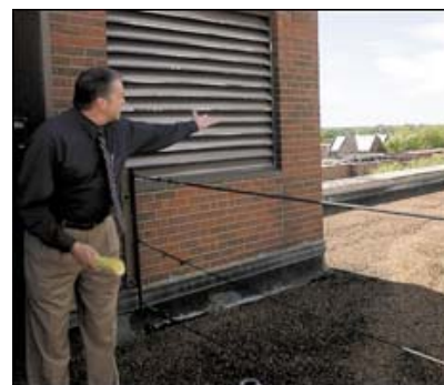
Katie Stockstill/The Morning Sun Paul Stewart, director of facilities planning for Pittsburg State University, stands on the roof of Heckert-Wells Hall Wednesday afternoon to show the building's sagging and leaking roof.
